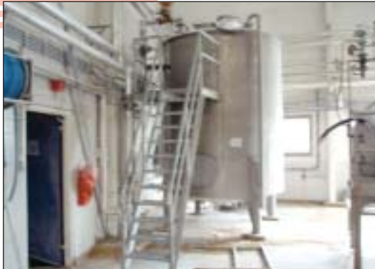
Ss tank with course way, pneum. stop valves, 2 feeding pumps, etc.
