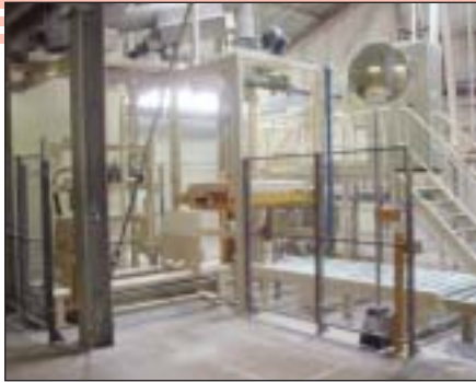
DeLaere big-bag filling plant, cap.: ca. 6 ton/h., with Siemens Simatic OV 7 operator panel, weighing unit: max. 1.500 kg.
