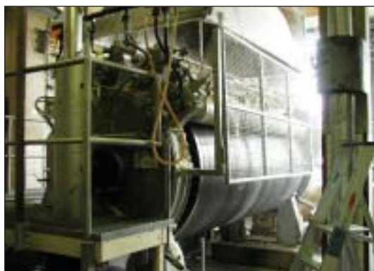
GMF rolling mill dryer, power cap.: 55 kW
