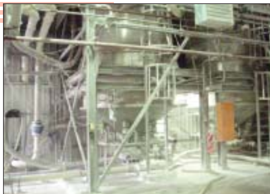
Dietrich Reimelt KG stainless steel silo (50-T-04), on weighing indicators
