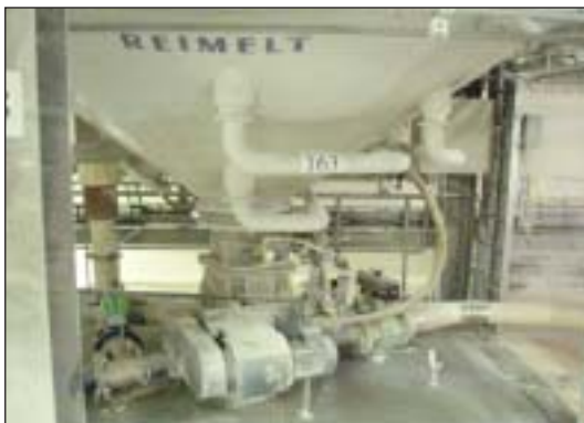
Reimelt ss bulk silo (50-T-12), full cap.: ca. 80 m 3 , with air valve, etc.
