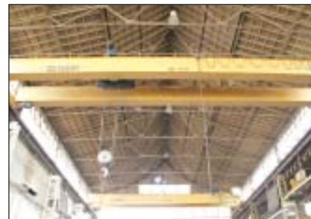
2 x GMK overhead crane, cap.: 25 tons
