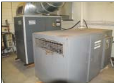
Atlas Copco Air Compressors
