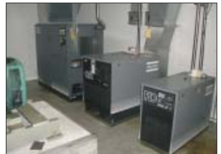
Atlas Copco schroefcompressoren met vriesdrogers / Atlas Copco screw compressors with freeze dryers
